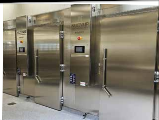
Zentralküche Care-Catering | INDUSTRY-LINE N300T2
